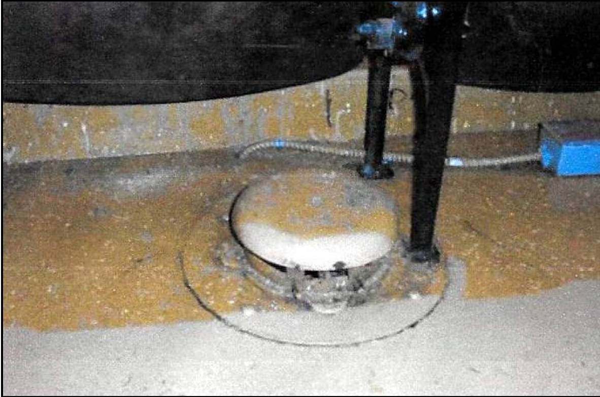
Supply air mushroom outlet under auditorium seats
