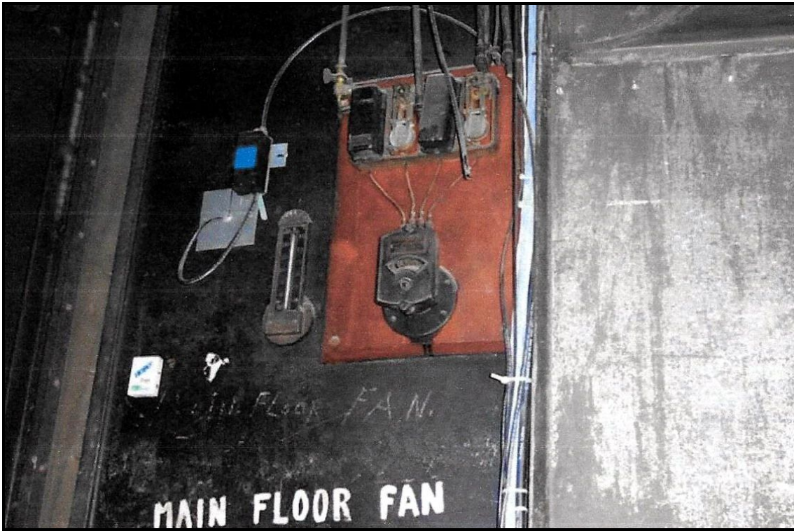
The Johnson 4-stage controls for the main supply air
